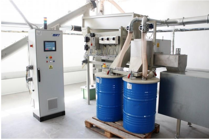
Figure 9.3. The equipment for mercury-containing waste processing line in "Bodnarivka" is the Swedish company "MRTSystemAB"
